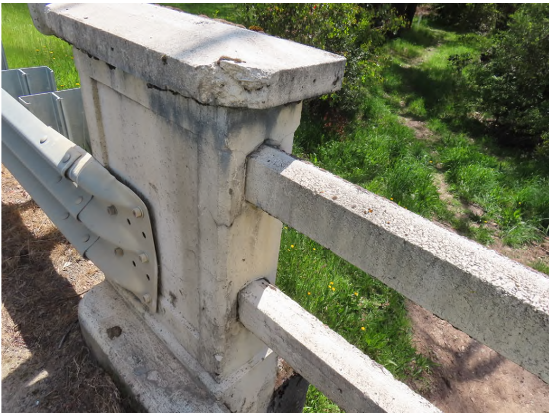
Photo 4. Minor damage to bridge rail post with some cracking.
