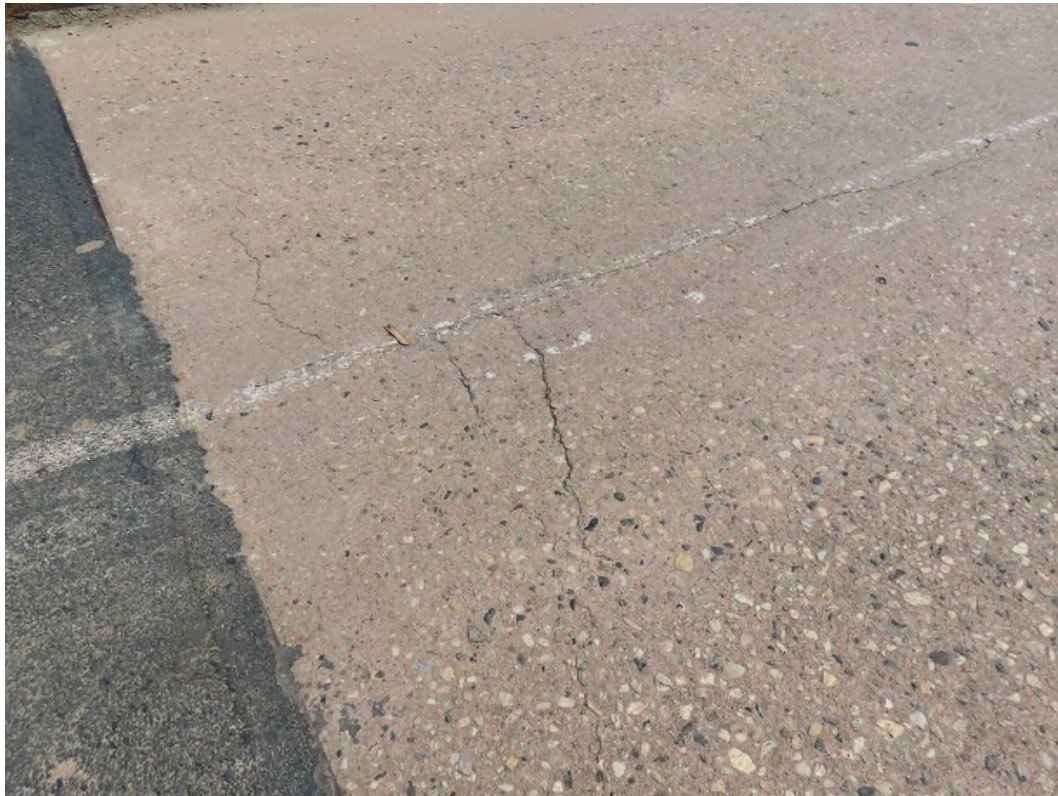
Photo 18. Transverse cracks in deck near east abutment.
