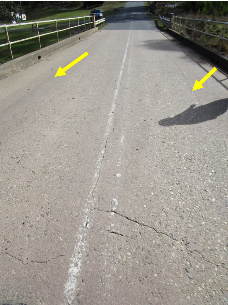
Photo 17. Transverse cracks in centre portion of deck. Note longitudinal construction joints (arrowed)
