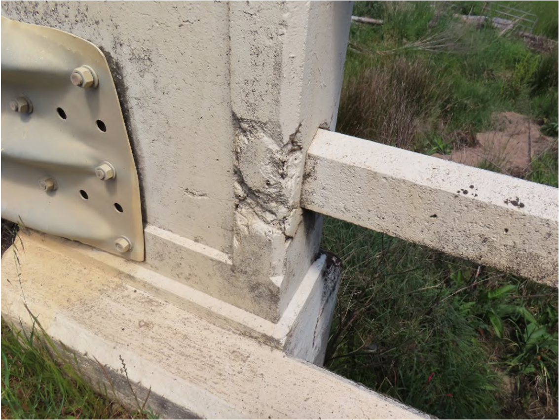
Photo 5. Minor damage to bridge rail post.
