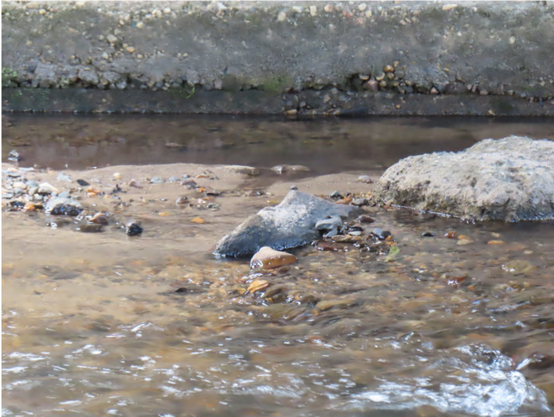
Photo 19. West span showing slight exposed footing under abutment.
