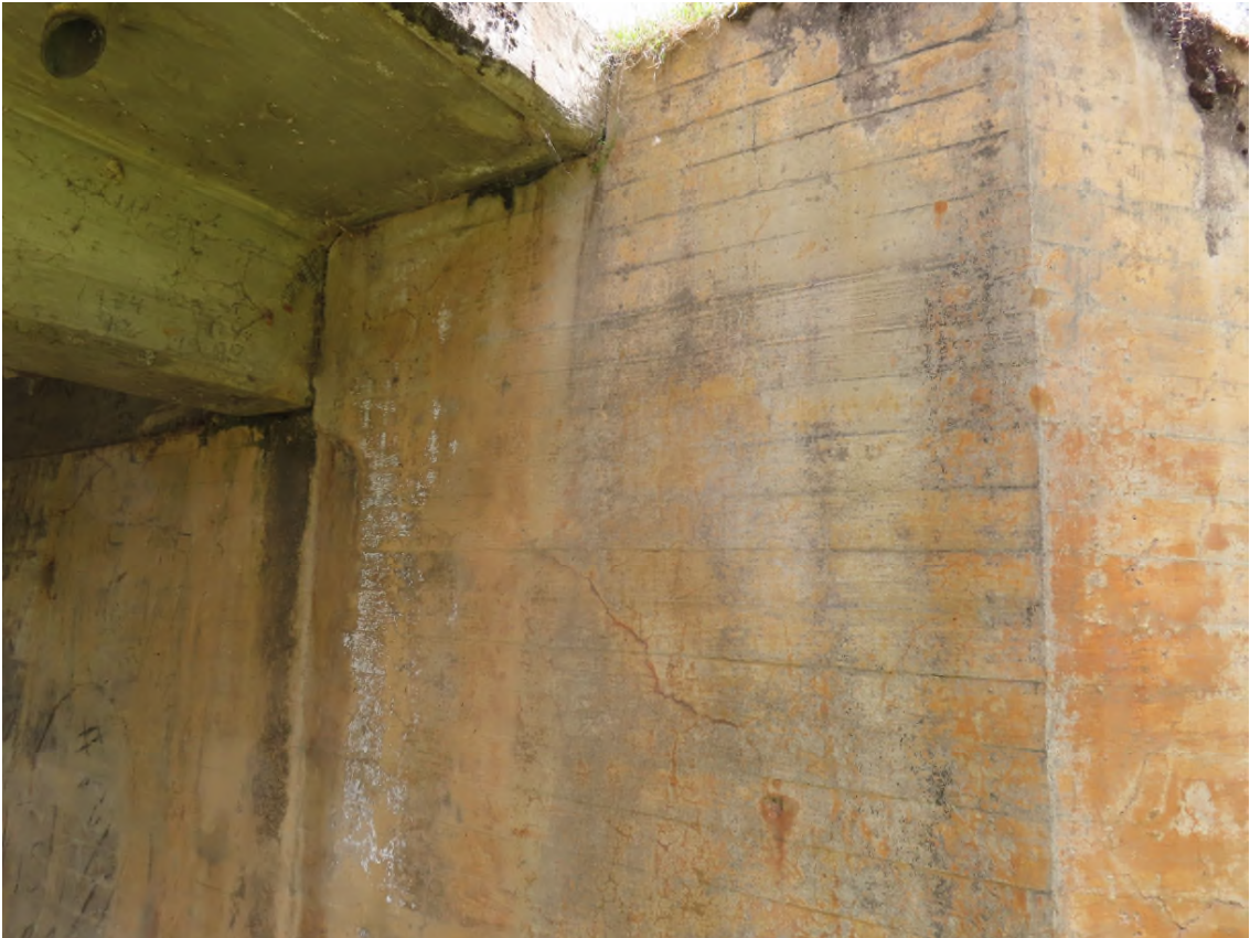
Photo 12. Typical crack in wingwall/abutment
