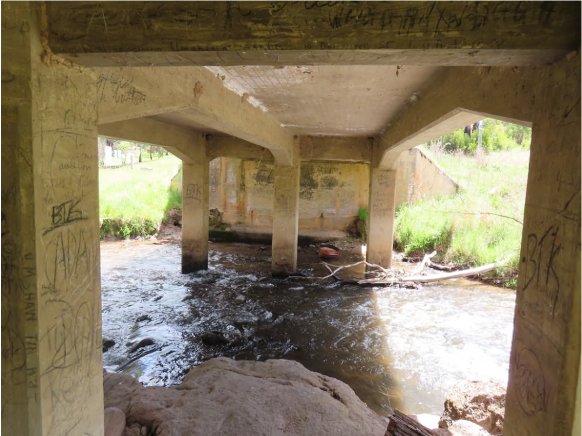
Photo 11. Underside of bridge. Note flood debris at pier.
