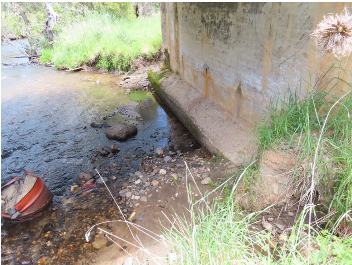
Photo 20. West abutment with slight erosion.
