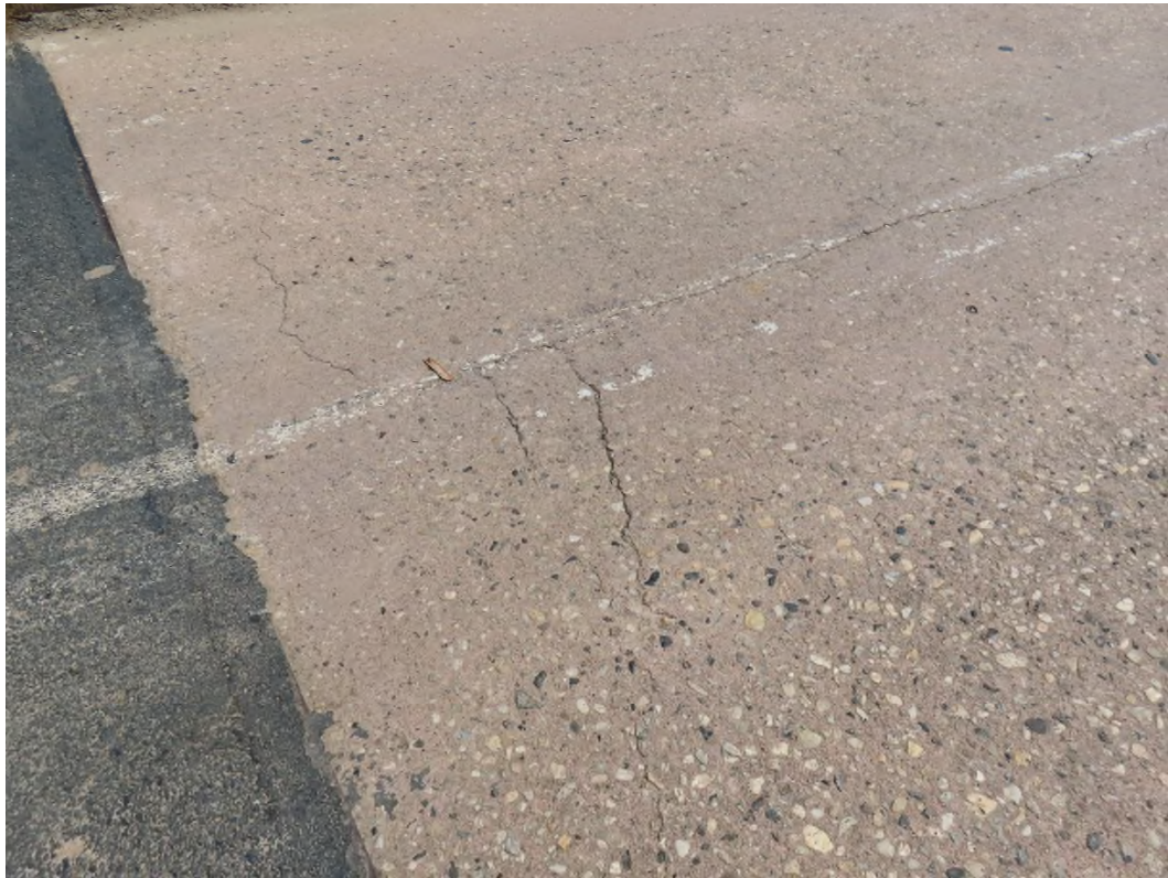
Photo 18. Transverse cracks in deck near east abutment.
