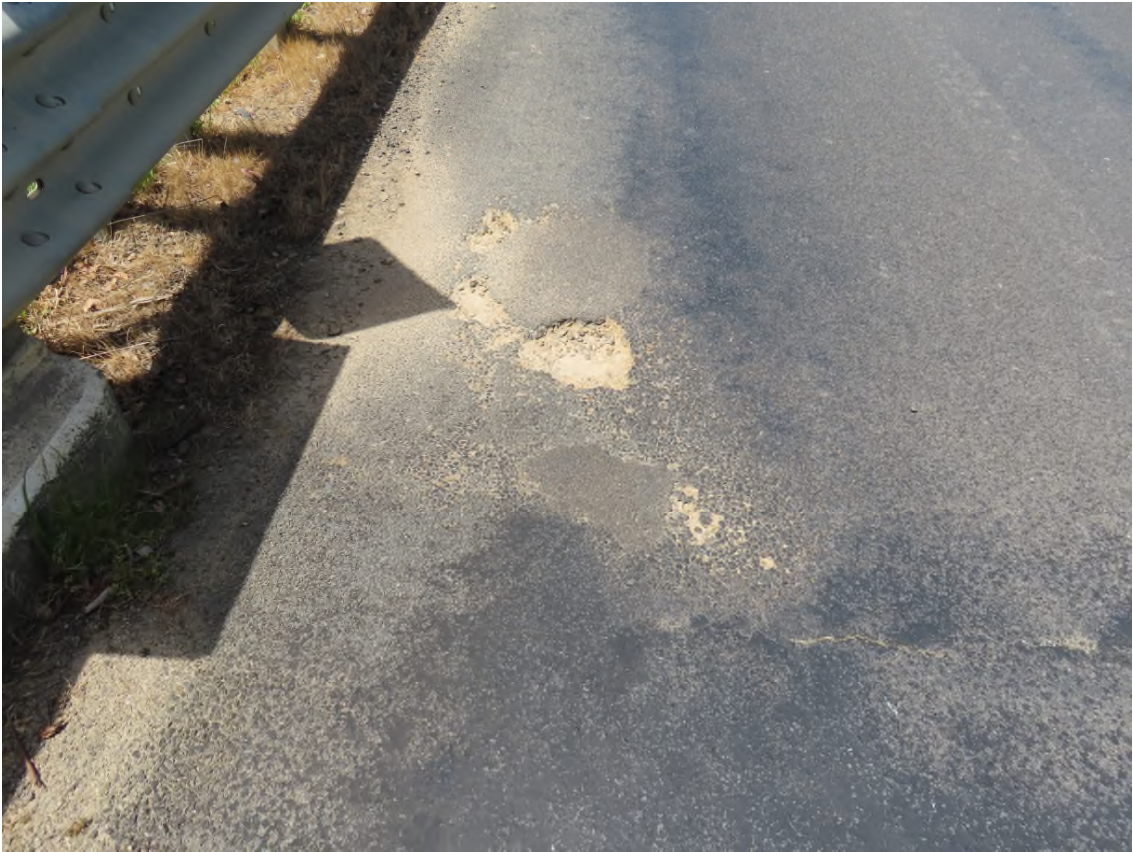
Photo 6. Pot hole at end of deck in road surfacing east end, north side.
