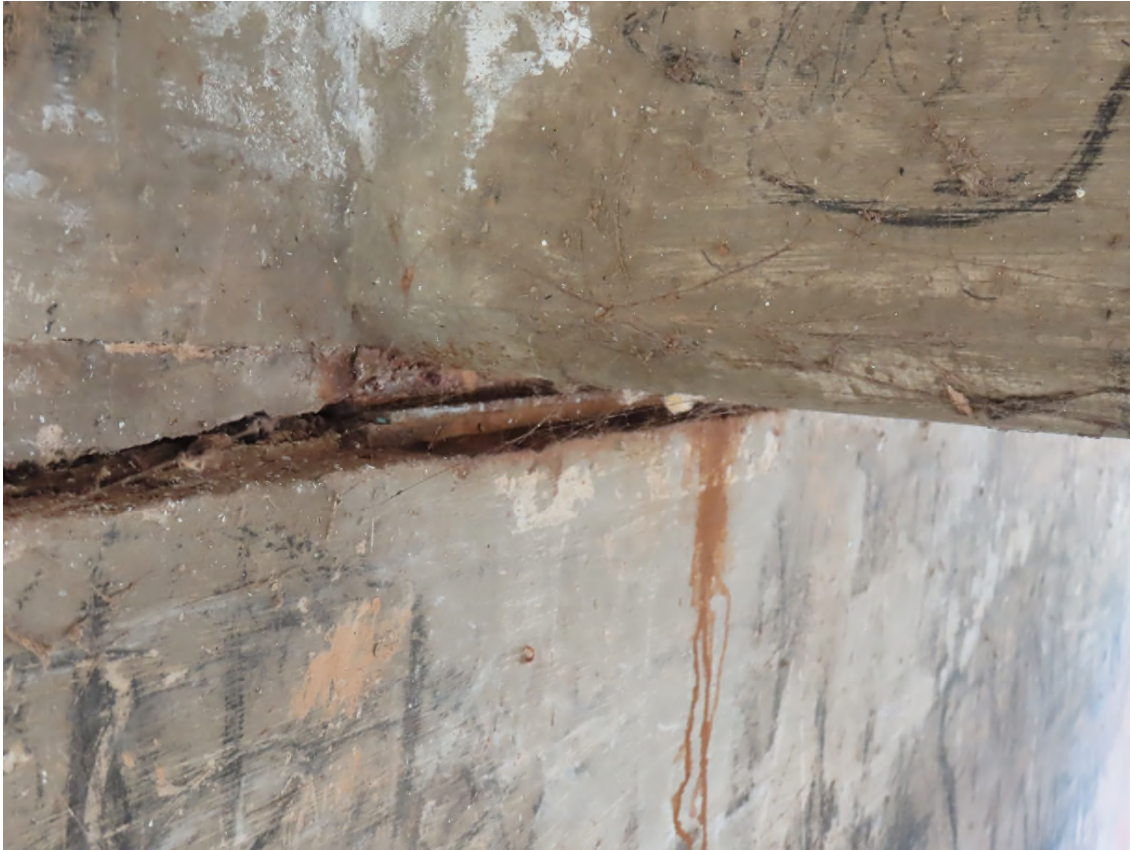
Photo 13. Tooma abutment (east end) bearing. Note on WAE drawings as a “fixed” abutment.
