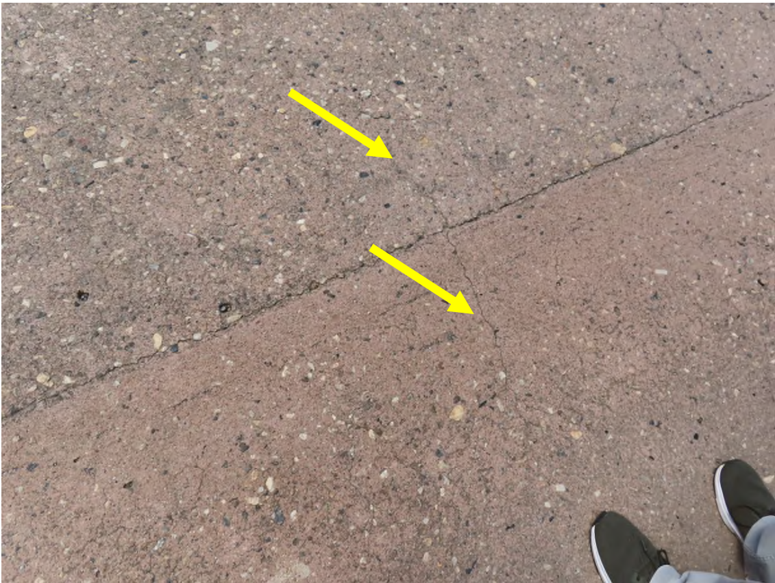
Photo 16. Transverse crack (arrowed) and longitudinal construction joint in deck
