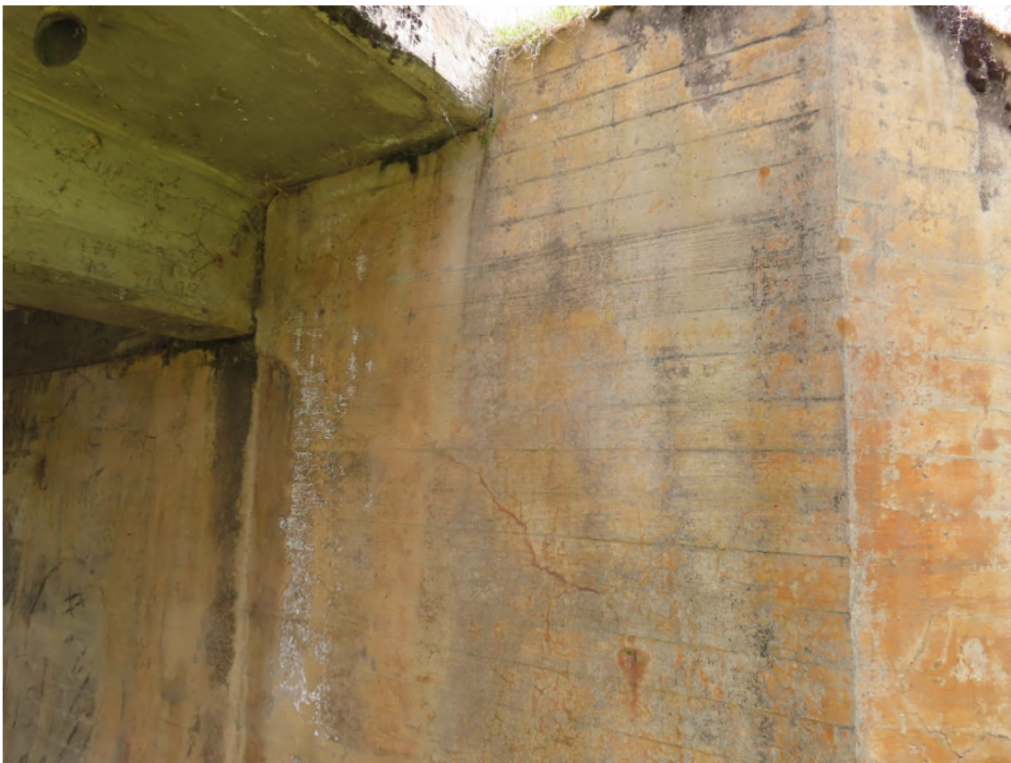
Photo 12. Typical crack in wingwall/abutment
