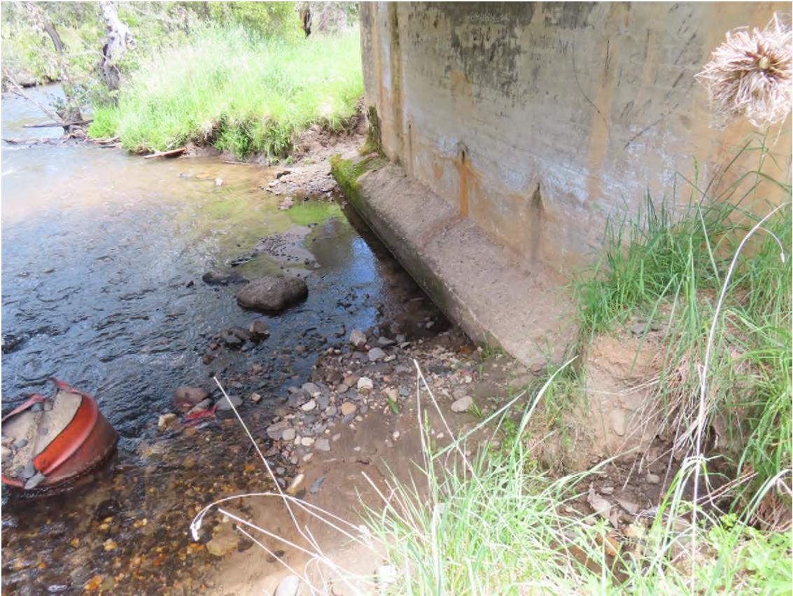
Photo 20. West abutment with slight erosion.
