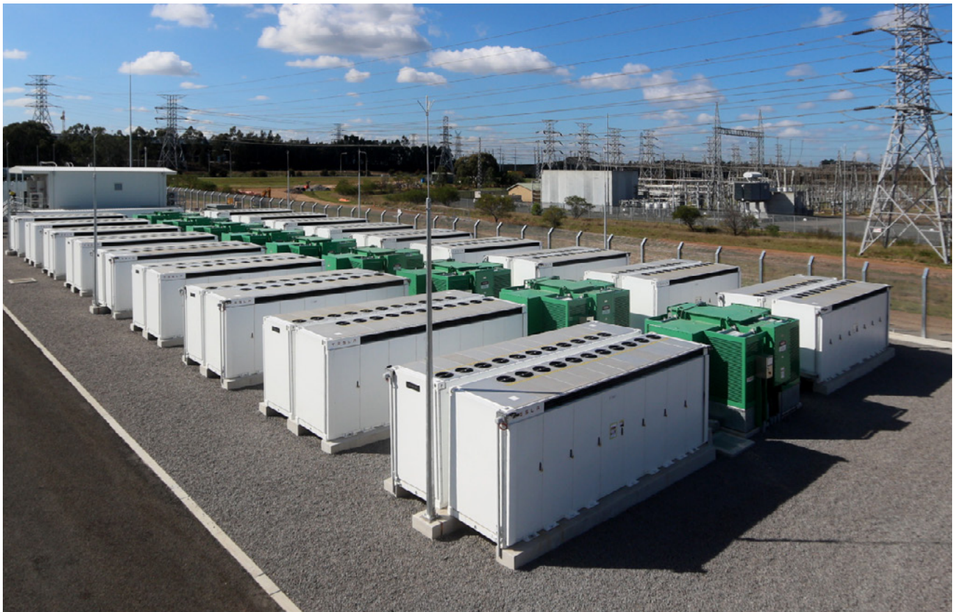
Photo 2 – Wallgrove Grid Battery looking towards Sydney West substation
